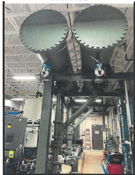
FIGURE 2-6: RAW WATER STORAGE
