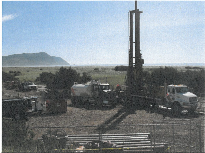
Chris Hyatt of HGS designed existing City wellfield
